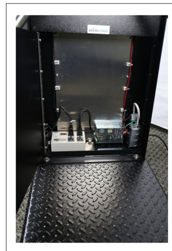
INSIDE: 4 outlet surge protector, DC fan for power supply
