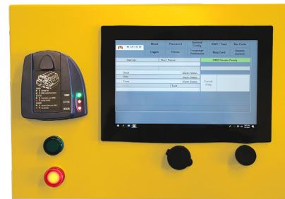
RWP Swing Gate Monitor
